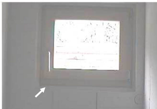
Figure 25 Utility Window – Visible
